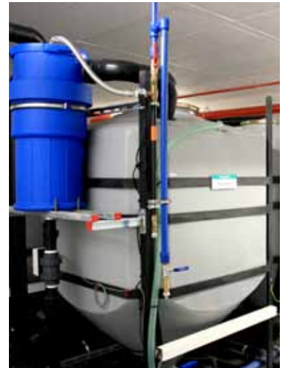
ABSA TOWERS WEST, JOHANNESBURG: 5 Star Green Star SA - Office v1 As Built Grey water system
