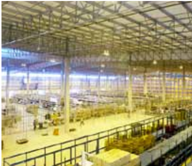
WOOLWORTHS DISTRIBUTION CENTRE, MIDRAND: The Building Management System is programmed to switch lights down to 50% when sufficient natural lighting is available.
